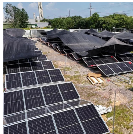
Masdar , Solomon Islands - Solar PV Plant in Honiara
