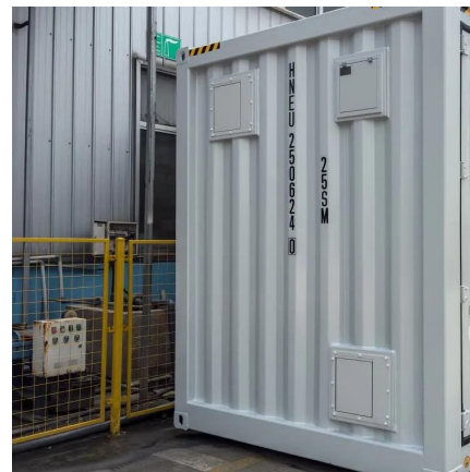
Uninterruptible Power Supply (UPS)
