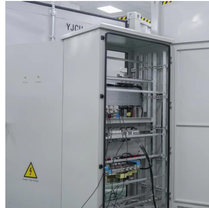
containerized battery storage , SUNTON POWER
