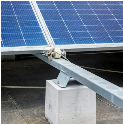
Solarcontainer: The mobile solar system
