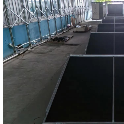
Solarcontainer: The mobile solar system
