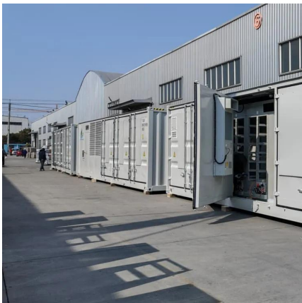
South tarawa energy storage
