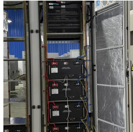
Official solar grid-connected power generation ...
