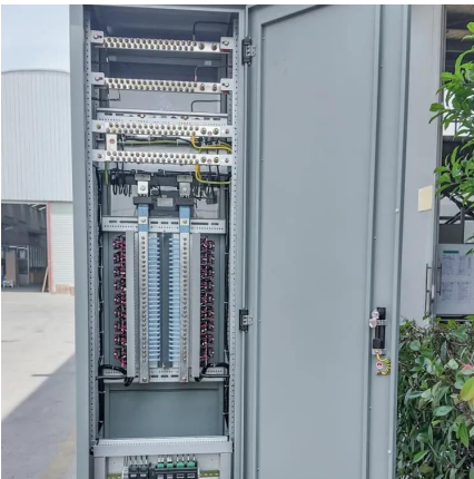
30 kW Solar System Hybrid (30kWh)
