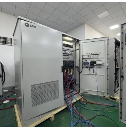
Mobile solar container
