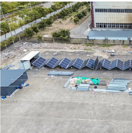
2MWH Containerized Solar Battery Storage System
