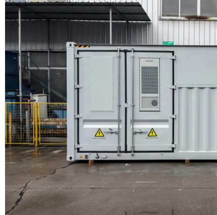
Container Battery Energy Storage Systems: Powering the ...
