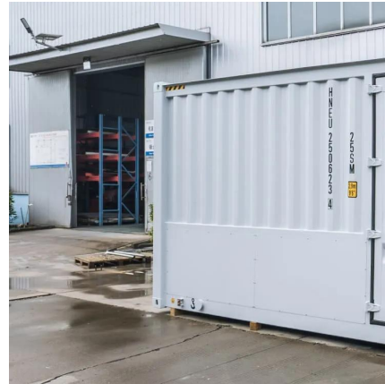
Power distribution box-GRL
