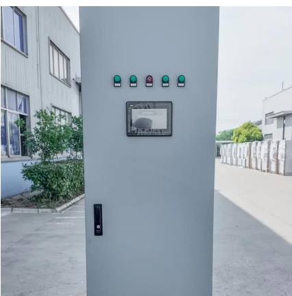
Energy Storage & Wiring Solutions in Kuala Lumpur: ...
