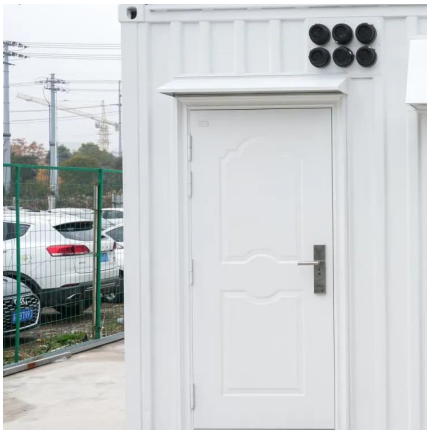
Kiribati: 500kW Solar PV & Water Protection
