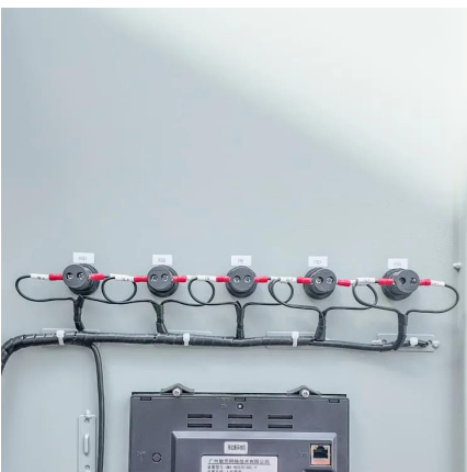
Fold-Out Solar Container Battery System Mali
