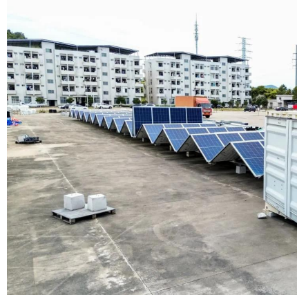
Photovoltaic energy storage power station Khartoum
