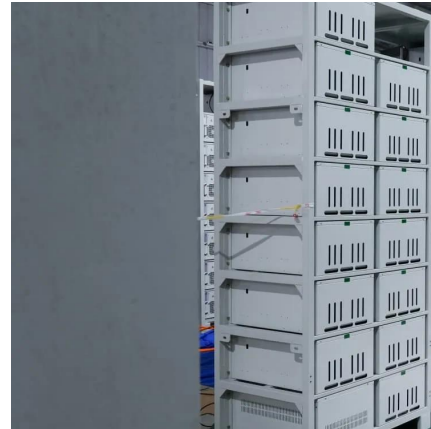
30kw Battery Energy Storage System
