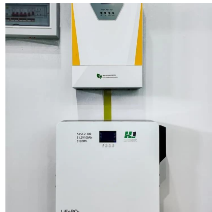
PFIC30K64P30 Foldable PV Container , 30kW/64kWh Solar ...
