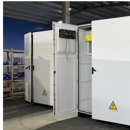
Battery Cabinet System
