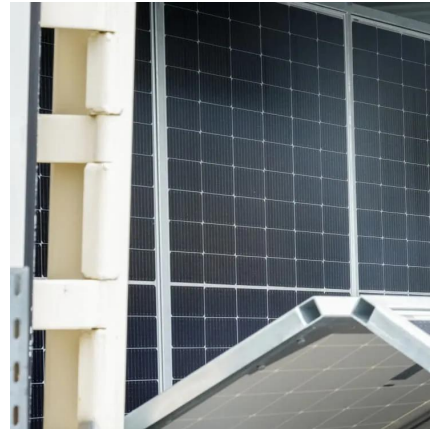
2kWh Vestwoods Power Station in Kenya
