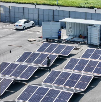
Energy storage container, BESS container.
