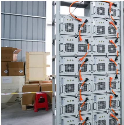
Solar-powered charging station
