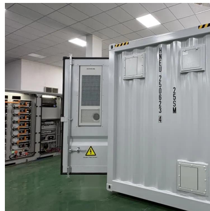
250KW 500KWH Container Battery Storage
