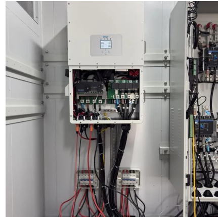
Solarcontainer: The mobile solar system
