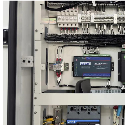
Energy storage system of communication base station
