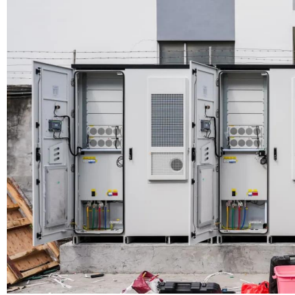
Solar Installation Company Boston MA , Viridis Energy
