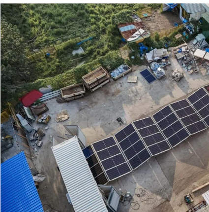
Battery Cabinet System
