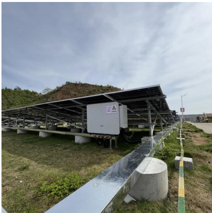
Battery Cabinet, Battery Storage ...
