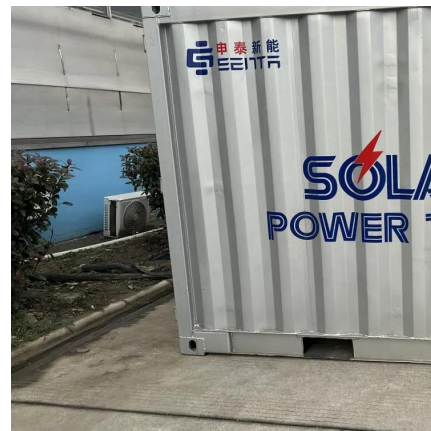
How to design an energy storage cabinet: integration and ...
