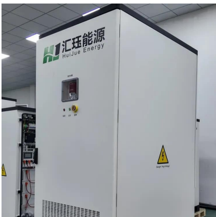
Certo C1 Battery Cabinet
