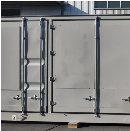
Base Station Lithium Replacement , Huijue Group E-Site
