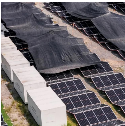
Energy storage container, BESS container.
