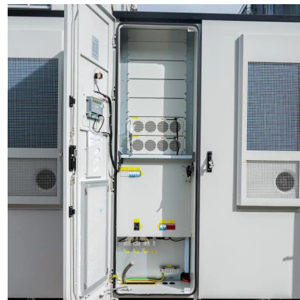
Battery energy storage system (BESS) ...
