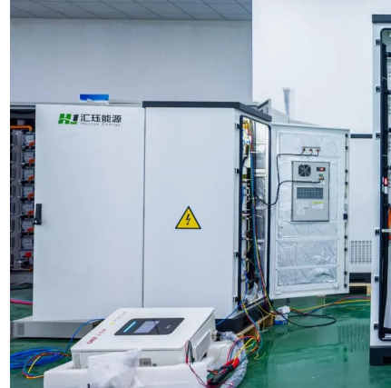
Off-grid container power systems
