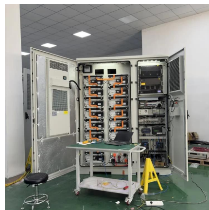
2MWH Container Solar Battery Storage System - Polinovel
