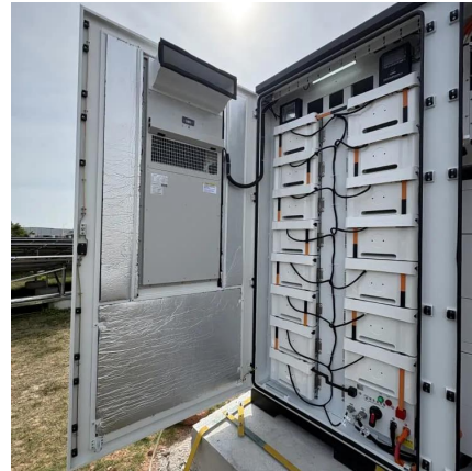
2MWH Containerized Solar Battery Storage System
