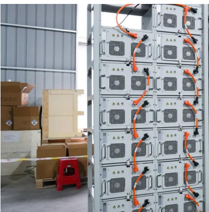
Solar Battery Cabinet
