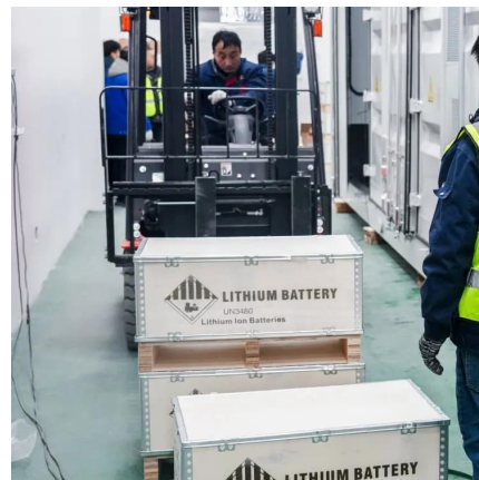
5MWh Containerized Energy Storage System
