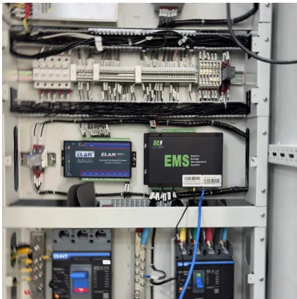
VIENTIANE NEW ENERGY STORAGE INDUSTRIAL PARK ...
