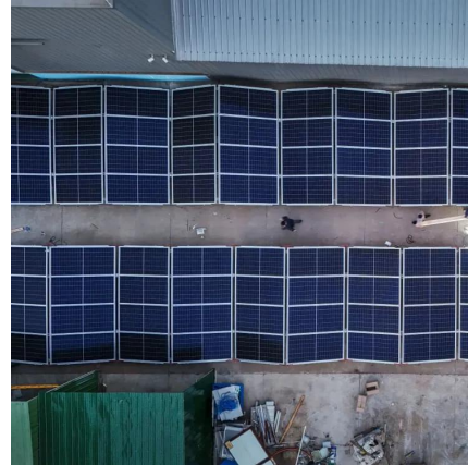
372kWh Battery Storage System
