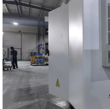
20FT Container 250KW 803KWH Battery ...
