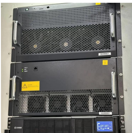
Container Energy Storage System
