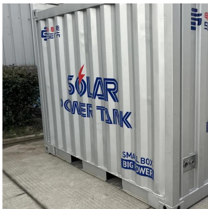
Dawnice 200kWh Battery Storage Systems
