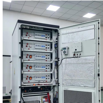
Solar Inverter, Solar Charge Controller, Off ...
